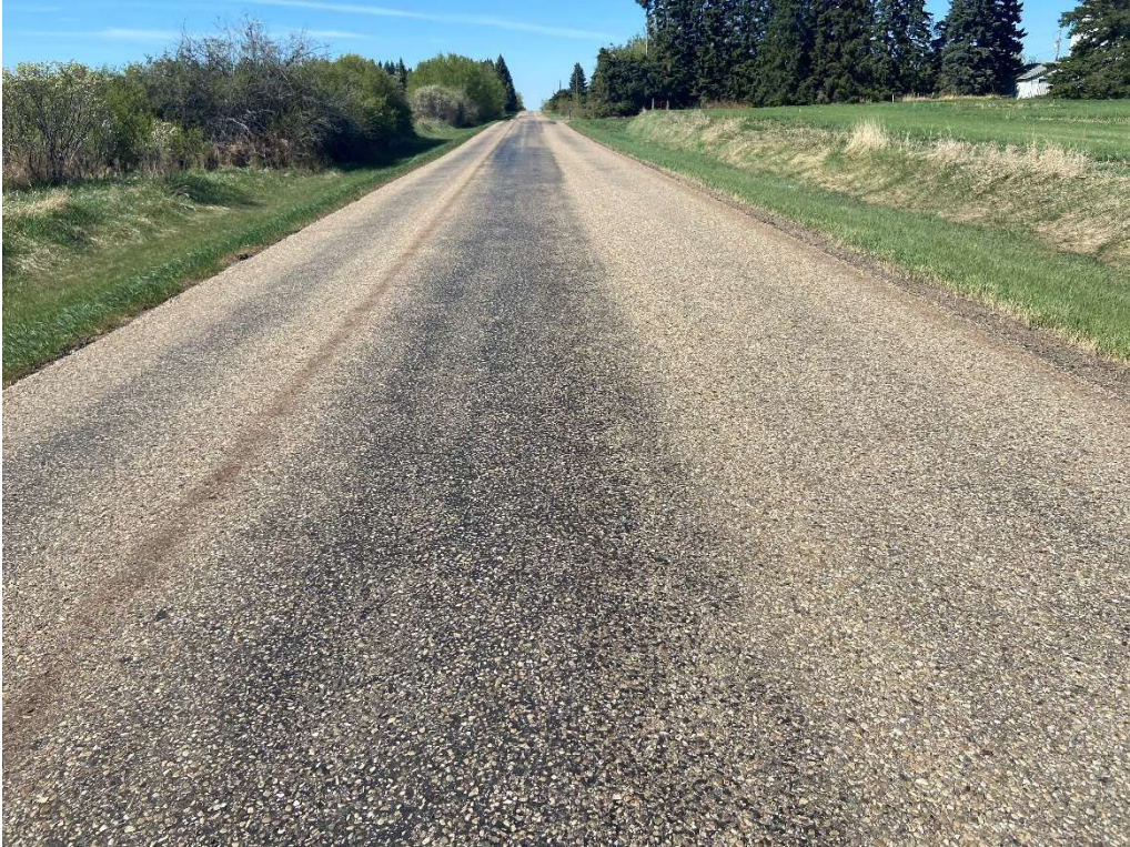
Class II road with old cold mix surface
